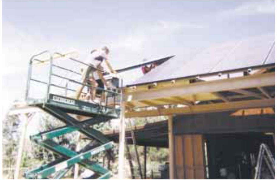
The PV array almost completed. Proper planning and attention to detail assured that everything went together without a hitch.
