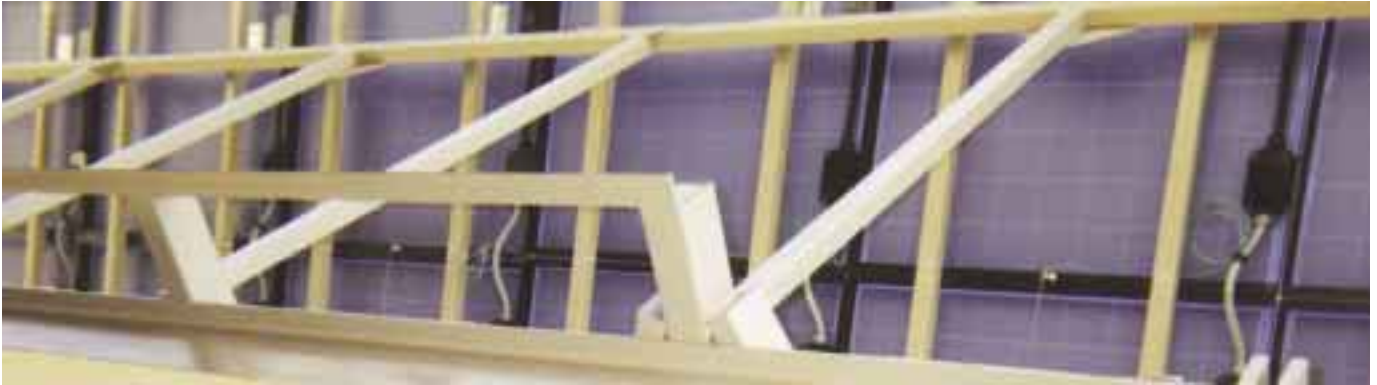
Underneath the completed array, the installation is tight and professional. Note the stout rack built by the author.
