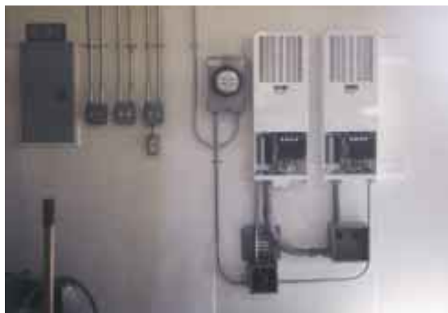
The ST2500 inverters feed RE to the utility grid.
