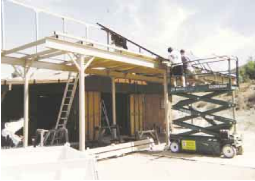
After installing the first few subarrays, it became second nature. Sheets of plywood kept the scissors lift from bogging down in the dirt.
